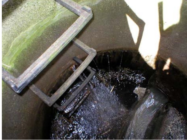
Figure VII-6 - Active Infiltration at Manhole GW18
